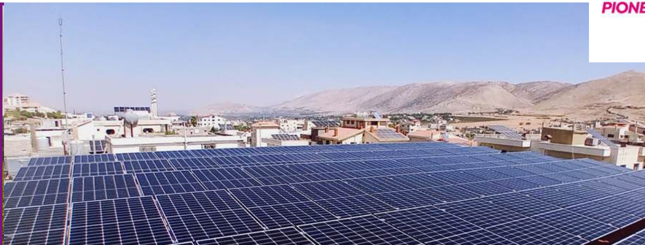
Largest solar system Aid Pioneers have installed in Lebanon so far (110 kWp)
